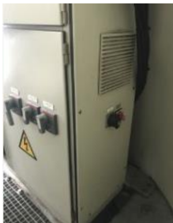
Lateral del armario ground, zona donde se ubica el seccionador Q12 Side of the ground cabinet, area where the Q12 isolator is located.
